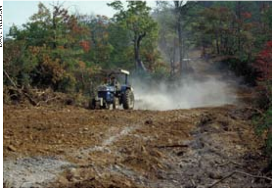
Cutting in lime with a tractor to improve soil pH in a linear opening (road).
