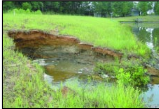
Poorly constructed ponds will result in failure.
