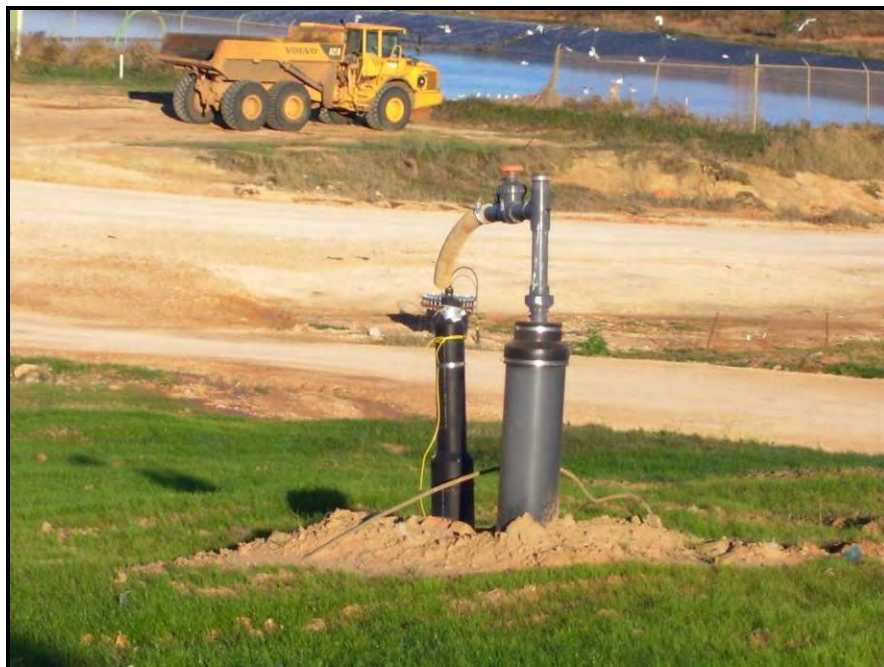
Seven (7) gas collection wells are drilled into the landfill waste and connected to the piping system leading to the flare.
