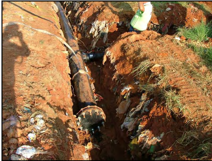
1,000 linear feet of piping is buried throughout the landfill. The piping system transports the gas to a flare where it is burned.
