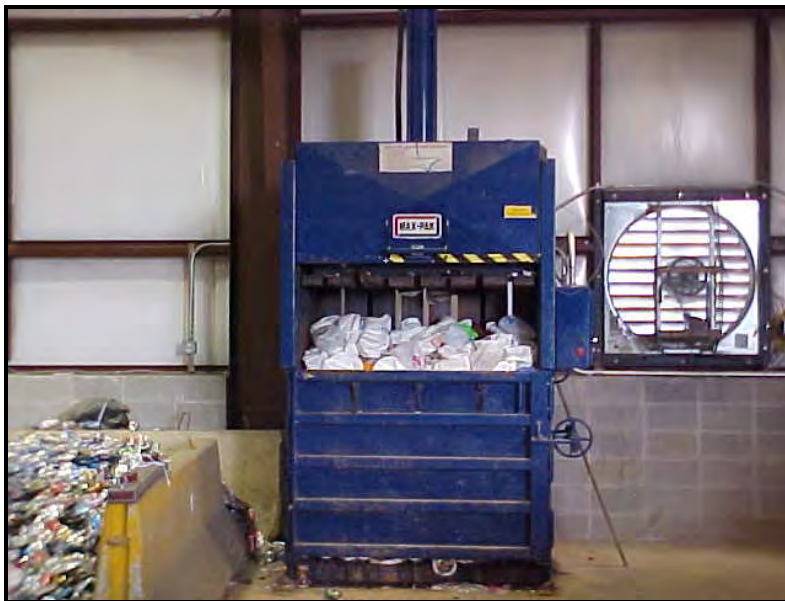
Vertical baler for baling plastic and aluminum; in FY 2007 14 tons of aluminum cans 18.3 tons of #1 plastic, and 16.3 tons of #2 plastic were recycled.
