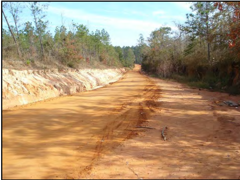
Barrineau Park Road - Approaching Perdido River Right shoulder ditch is filled with sediment.
