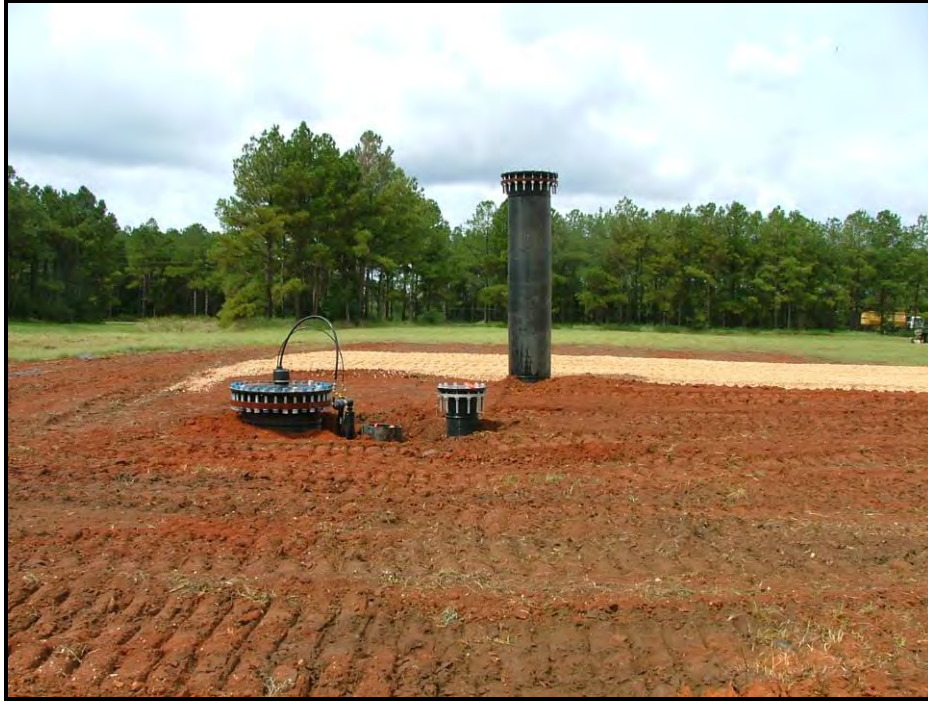
A landfill flare will be connected to the piping system shown above. Burning the landfill gas will reduce NMOCs by 98 percent.
