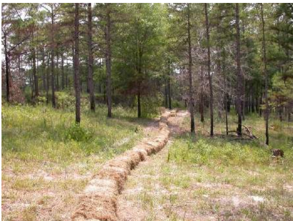
View of completed hay bale pen along west side of enclosure looking south.
