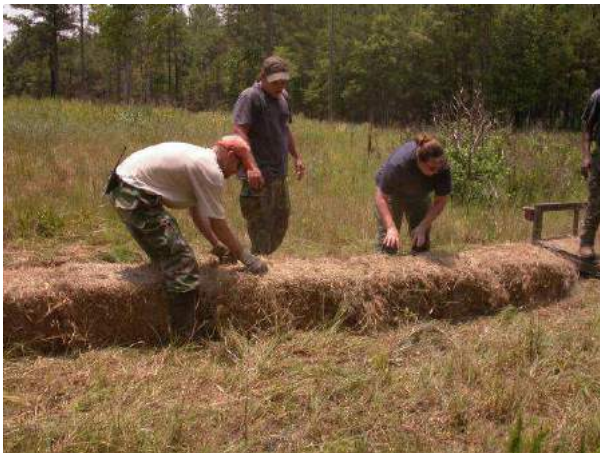
Placed hay bales being pulled tightly together to eliminate gaps between them.
