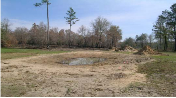
Picture 4: Construction of an ephemeral pond for amphibian habitat (Photo Credit: Mark Bailey, 3/8/06).
