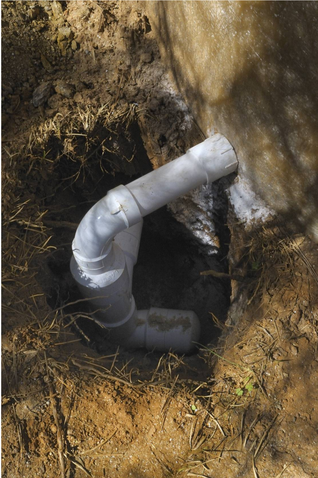
Figure 25. PVC refugium set in place extending 76-91 cm (30-36 in) underground. Hole surrounding the refugium is filled with soil once refugium has been set in place and secured to the tub.
